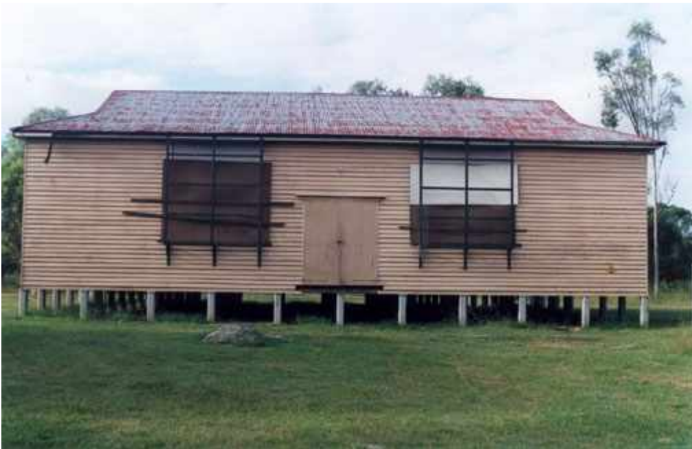
Sandgate Drill Hall moved to its new site -note elevation and replacement concrete stumps (February 2000)
